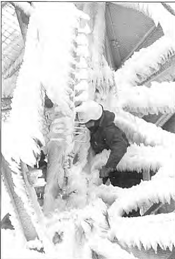
A rigger is clearing snow from a yagi antenna. This photo illustrates the "flag ice" phenomenon and the impact it can have on both the tower and the antenna's attached to towers. (Photo courtesy Ian Greaves Telecom)
