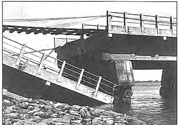
1931 Hawke's Bay Earthquake. Lateral spread of the embankment has allowed the landspan to drop off the first pier support collapsing it to the ground. The rail track has remained suspended free of the fallen bridge. (Photo Institute of Geological and Nuclear Sciences)
