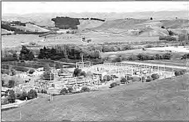
Redclyffe Substations for Transpower and Hawke's Bay Network showing proximity to the Tutaeakuri River.
