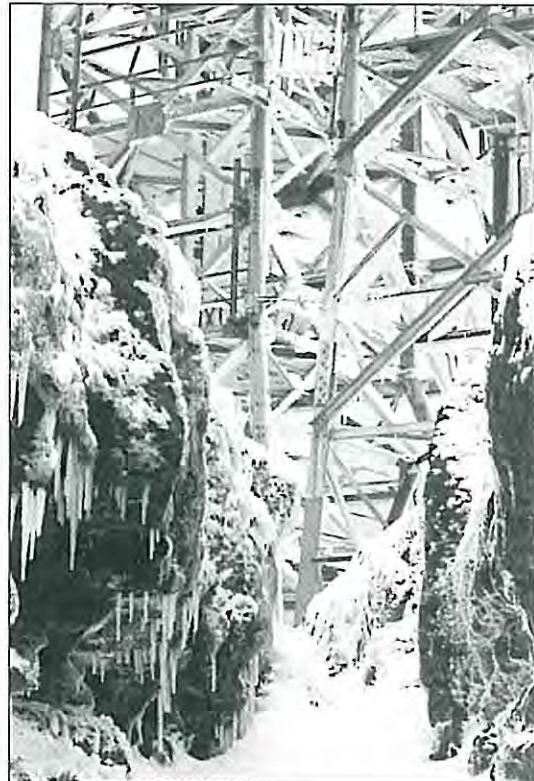
Snow and ice conditions at TeWaka Repeater Station taken from a perspective between 2 rock outcrops. At the time of this photo there were 2 towers on the site, the smaller one in the foreground has since been dismantled and removed. (Photo courtesy Ian Greaves Telecom)
