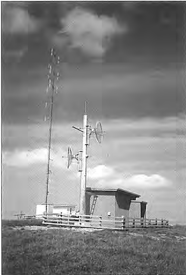
Rangitoto radio site, Transpower Hut and Discs Tower Hill (Photo courtesy Garth Cassidy)
