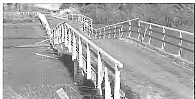
Flood damaged bridge at Makaretu, September 1988
