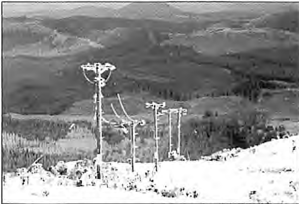
Power Lines feeding power to TeWaka have had their spans shortened by including extra poles. This was necessary to prevent the combination of ice and wind causing the spans to collapse under the strain. (Photo courtesy Ian Greaves Telecom)
