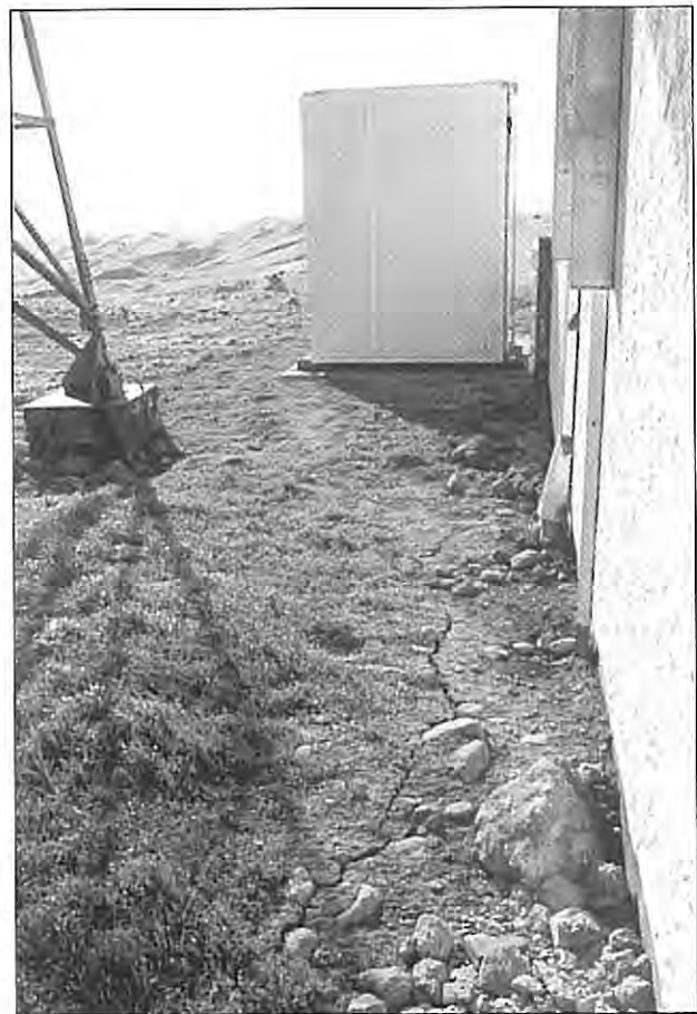
Photo taken on the North side of Takapau Microwave Radio Station after an earthquake event which occurred during the mid 1980's. There is evidence of backfill settlement around the foundations of the building and tower footings. (Photo courtesy Ian Greaves Telecom)
