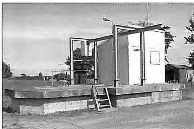
Fitzroy Street pump station which is the final pump station in the Wairoa system. At this point, the sewage is pumped into the wastewater plant. (Photo courtesy WDC)
