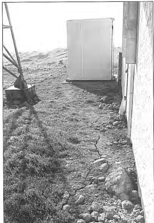
Photo taken on the North side of Takapau Microwave Radio Station after an earthquake event which occurred during the mid 1980's. There is evidence of backfill settlement around the foundations of the building and tower footings. (Photo courtesy Ian Greaves Telecom)
