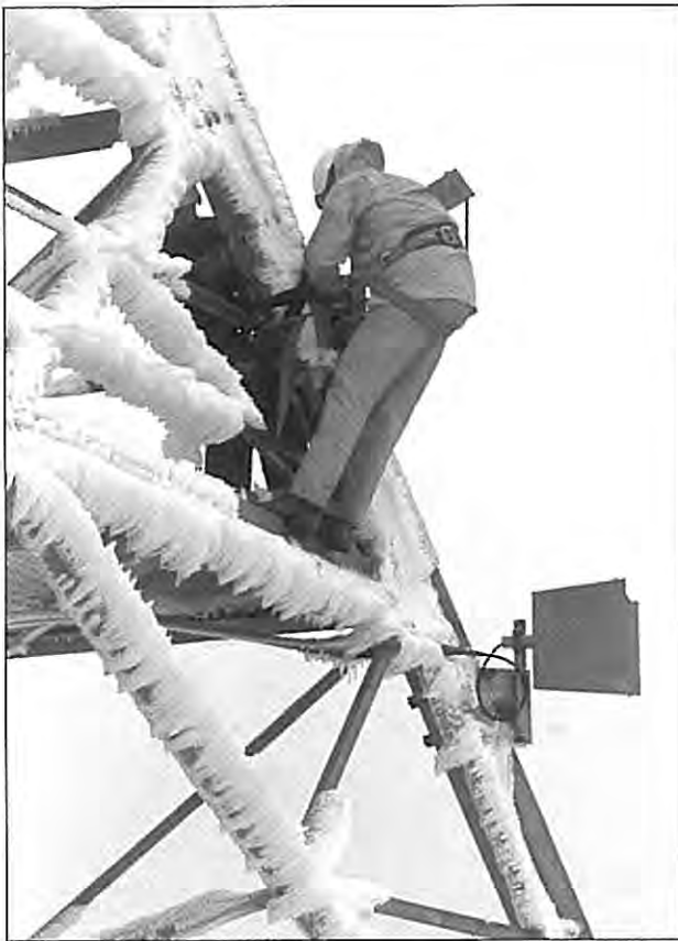
A rigger is clearing ice away from a corner reflector antenna on the Te Waka Microwave tower. The lower antenna has already been cleared of ice and should now be performing normally. The formation of "Flag Ice" on this structure is not uncommon. (Photo courtesy Ian Greaves Telecom)
