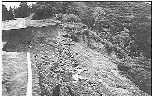
Landslip Mohaka Hill State Highway 2 July 1997 (photo courtesy Opus)
