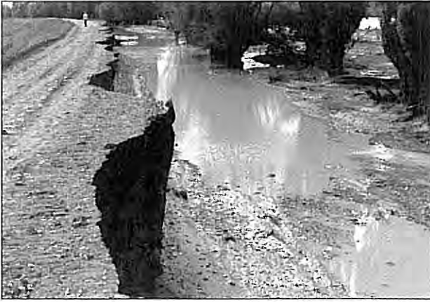
Ngaruroro River Stopbank with scour damage after Cyclone Bola 1988. (Photo courtesy HBRC)
