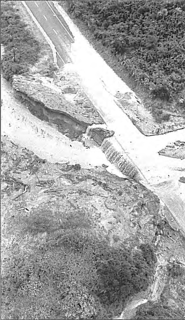
State Highway 5 Runanga flood 1985. (Photo courtesy of Opus)
